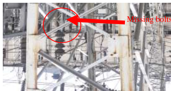
Figure -4 welded connection instead of bolts at Column A2 bay DT-1 feeder
