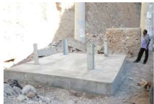
Figure 14: Block foundation covering all four legs of tower
