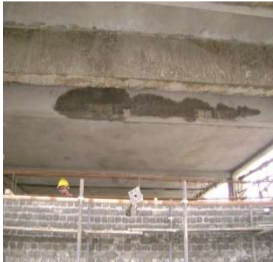
Figure 6C Water Leakage during Testing Work
