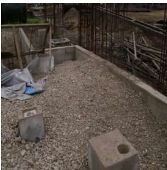
Figure 8 Gravel filling with small size in pit of transformer
