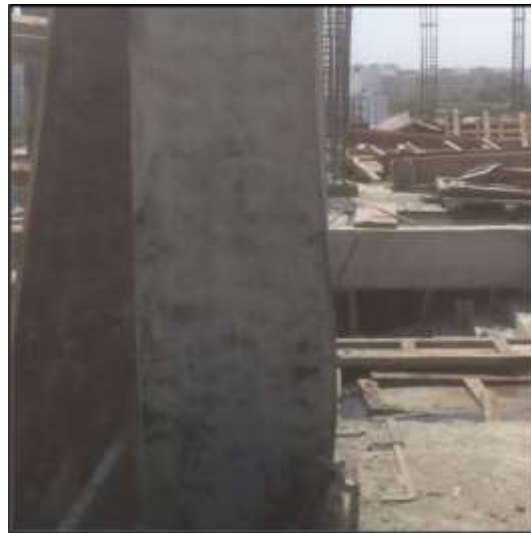
Figure 5 Building of finished Concrete due to weak shuttering
