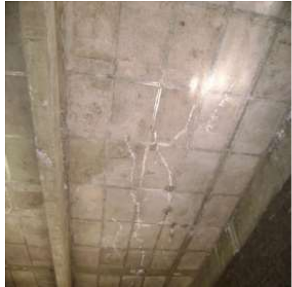
Figure 6D Water Leakage during Testing Work
