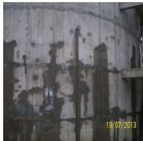
Figure 6B Water Leakage during Testing Work
