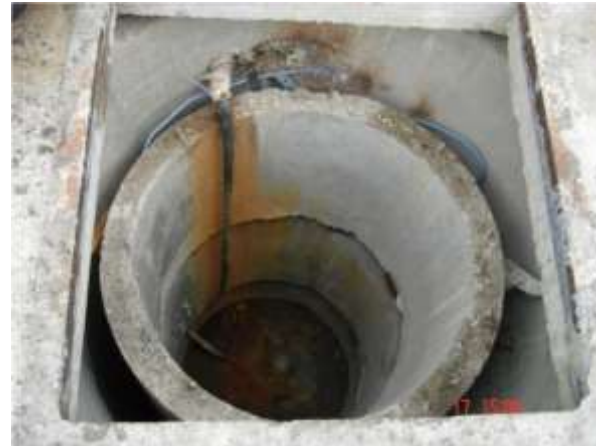
Figure 26 Electric well for setting concrete in precast foundation
