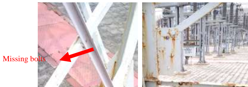
Figure -3 missing bolts at Column C4 bay D station
