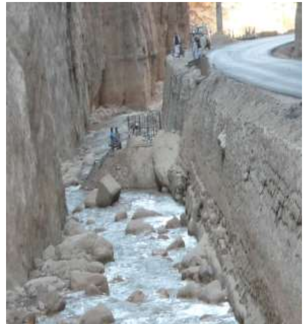
Figure 13: View of Narrow Road and water flowing canal where foundations had to be made
