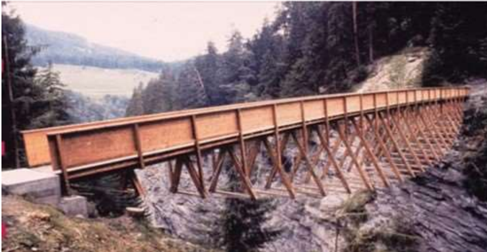
Figure 1: Traversing Bridge showing the use of locally available timber to enhance its sustainability.
