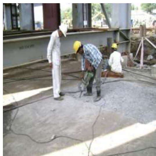
Figure 9 Concrete chipping not taken care of finished floor
