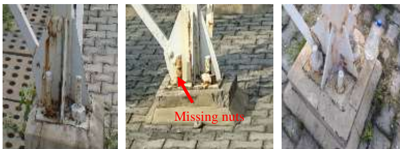
Figure 7 Missing nuts in foundation bolts in Column B4, B9 and C9
