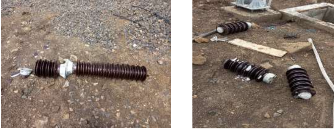
Image 2: Photographs of damaged equipment.
