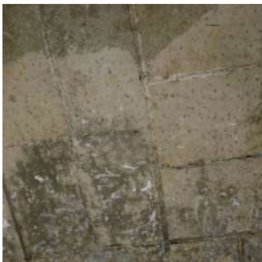
Figure 6A Water Leakage during Testing Work
