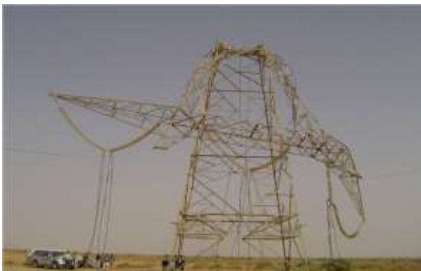
Figure 5: Damaged Transmission Line Tower
